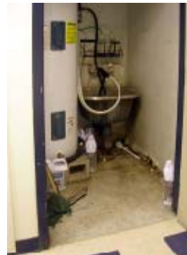
Water Heater 1 Hot Water-1
