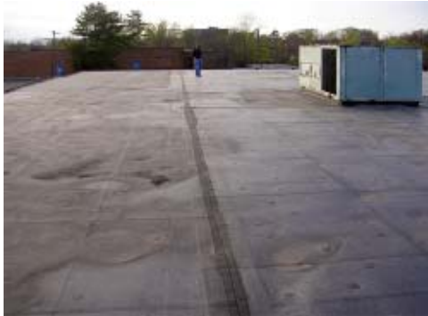
Roof 1 Roof Top Unit One
