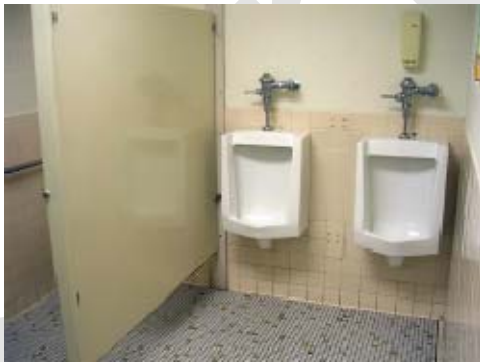
Toilet Rooms 3 Wall Mounted
