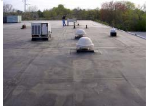
Roof 6 Exhaust Fans and DX Unit
