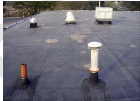
Roof 4 Vents & DX Unit
