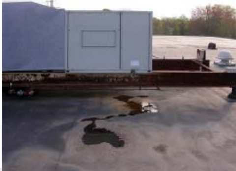
Roof 5 Roof Top Unit Two
